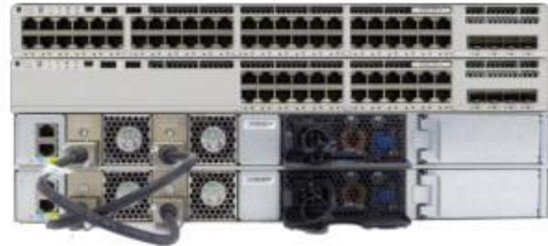
9200L Fixed Uplinks & Fans
